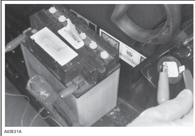
12-VOLT BATTERY PLUGGED TO BUZZER
