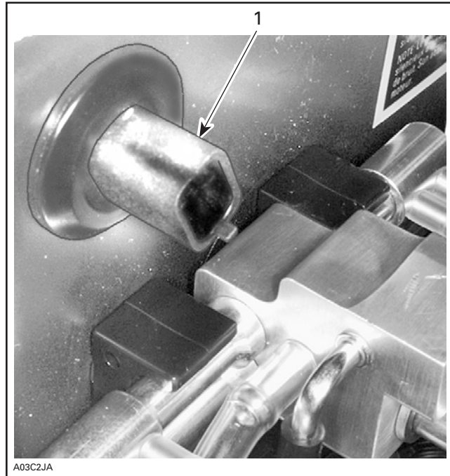
1. Air temperature sensor
